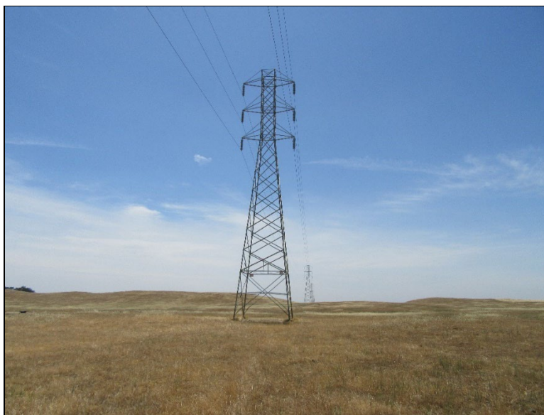
Figure 10. P-34-2195; Transmission Line Overview (view south; May 27, 2022).
