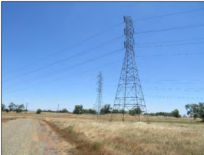
P-34-5267 and -5268; transmission line overview (view east; May 27, 2022).
